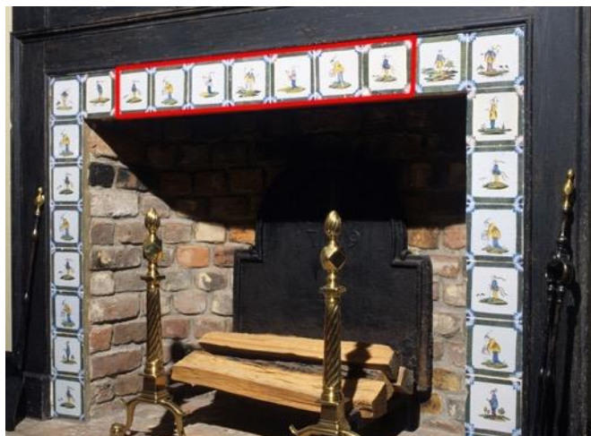
Figure 1. Bertrand fireplace, red rectangle shows the area where the plaster mounting material has become detached from the steel support beam.
