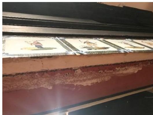
Figure 2. Detail of steel bar (red) and thick plaster behind the top row of tiles where it has become detached and cracked.
