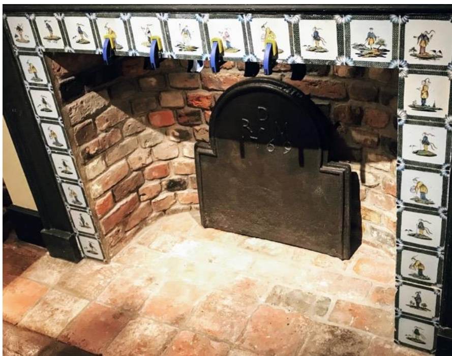
Figure 3. Top panel of tiles is clamped in place after injection of adhesive.
